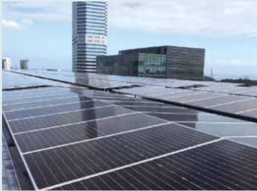
More solar panels were installed at MBC Block 20 during the year to harness solar energy
